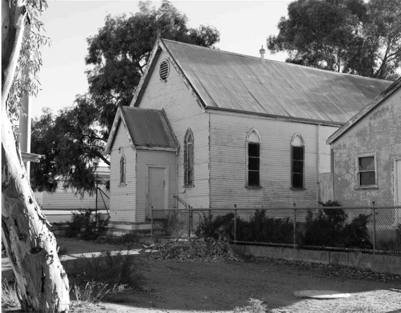
Figure 47 : Thomas Street Methodist Church building. Closed for many years and having had a range of uses the building forms part of a small local group of shops and church buildings but is at the point of collapse and is not recoverable. Many of the more minor church buildings have been lost.
