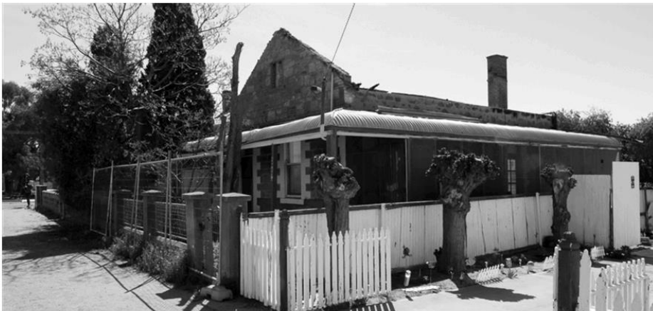
Figure 73 : An early stone house damaged by fire that is unlikely to be recovered.
