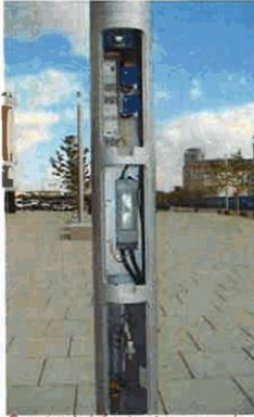
Smart pole infrastructure example
